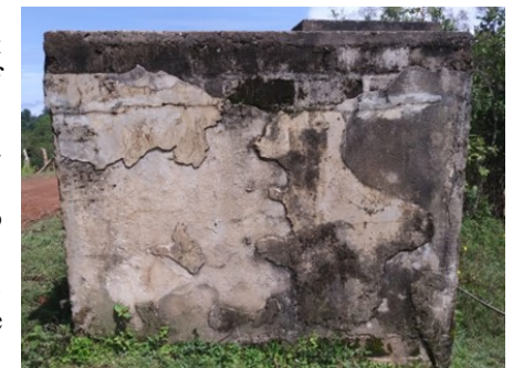
Deteriorating water tank
